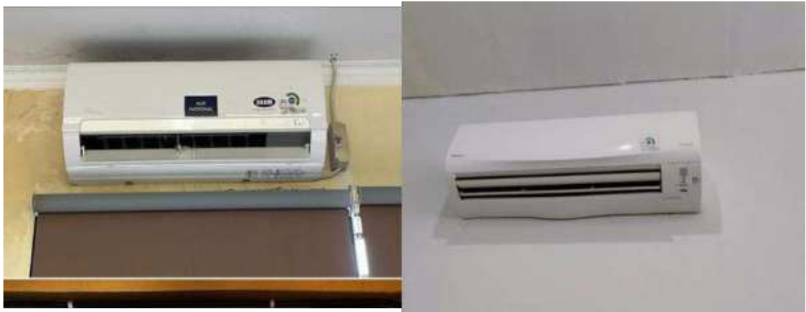
Gambar 4.8. Use of air conditioning system (AC) with inverter technology. Left: AC unit at the Faculty of Forestry; Right: AC unit main library
